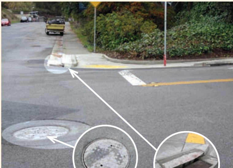
Sewer maintenance hole cover
